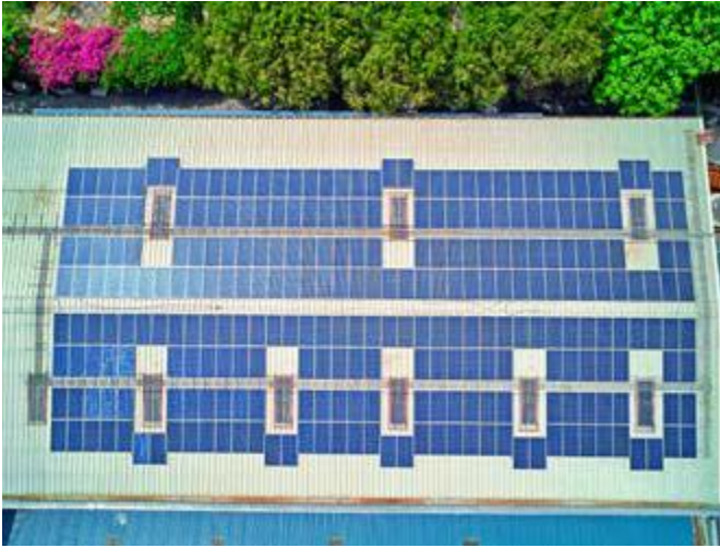
■ Rooftop Solar in Hapur Unit-1
