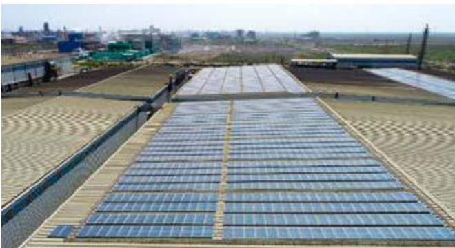
■ Rooftop solar system at Dahej unit
