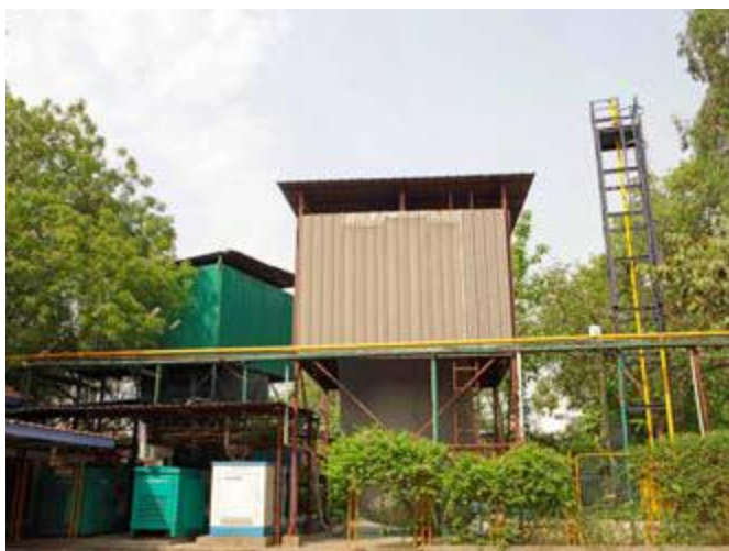
■ Biogas System, Hapur
