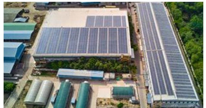
■ Rooftop solar system at Hapur II
