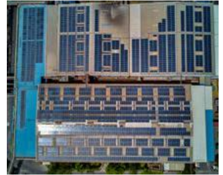
■ Rooftop solar system at Hapur Factory Unit I
