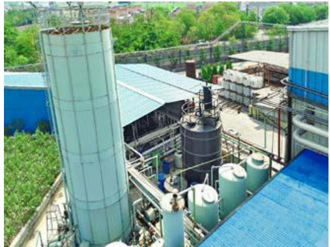
■ RO plant for water filtration & recycling in MIL, Hapur
