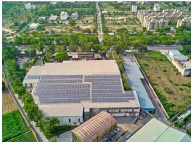
■ Rooftop Solar, Hapur
