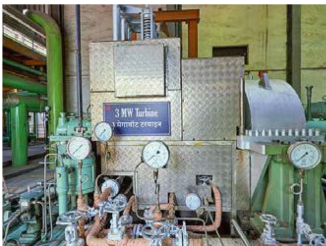
■ Biomass Based Turbine, Hapur
