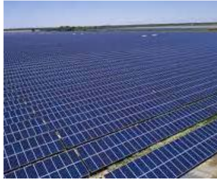
■ Ground mounted solar plant at Hissar
